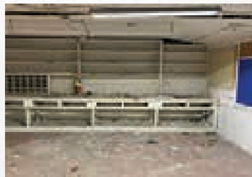
A room with debris left over from a rage room break session.
